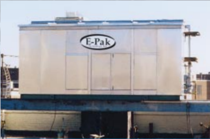
65 Unit Condominium Building, Phila, Pa Capacity 145 Tons with 44 degrees LWT @ 78 degrees F WB Air on the condenser
