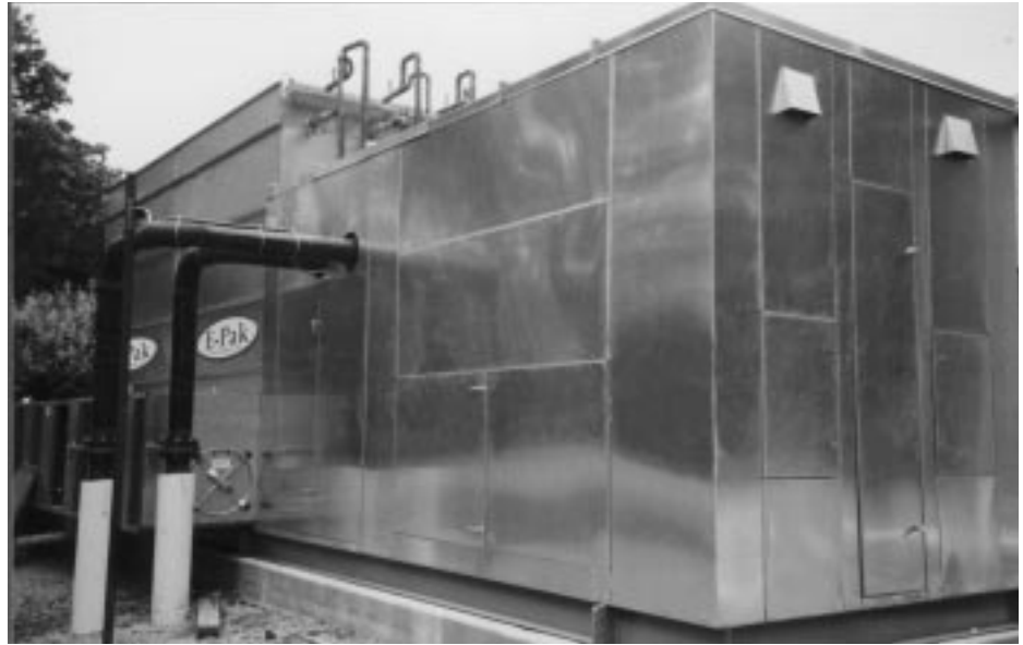
Princeton, New Jersey — 300 ton Chilled Water Plant with sound attenuation and plume abatement coil (hot gas de-superheat coil which runs the length of the condenser).
