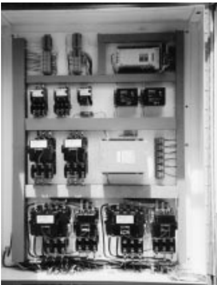
E-Pak Control Panel
