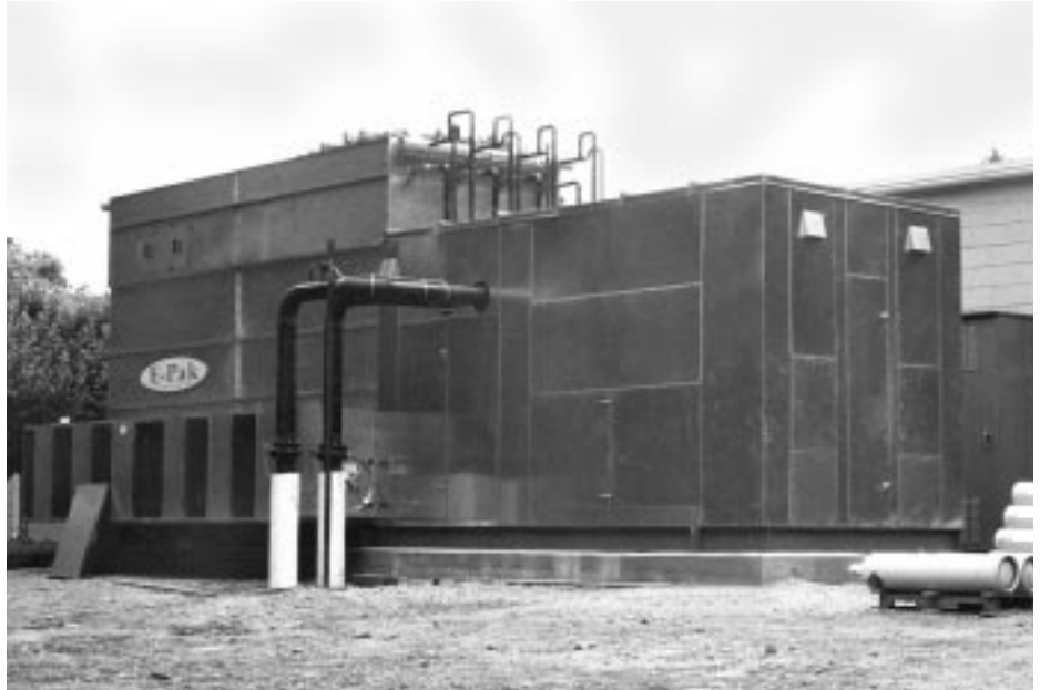
Princeton, New Jersey — 300 ton Chilled Water Plant with sound attenuation and plume abatement coil (hot gas de-superheat coil which runs the length of the condenser).
